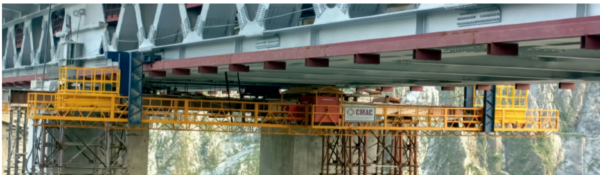
Self Propelling Maintenance Platform @ 331 Meters Height Horizontal Travel (290 Meters, 70 Meters, 80 Meters) Anji Khad River @ Jammu, First Cable -Stayed Railway Bridge in India
