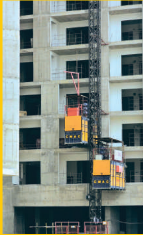
Passenger & Material Hoist (PMH)
