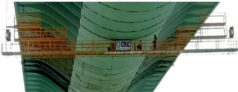
Special SRP for Anti Corbonation Coating (ACC) at Cable Stayed Bridge, Durgam Cheruvu, Hyderabad
