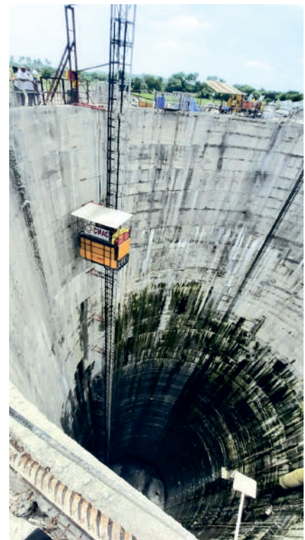
PM Hoist in Pump House
