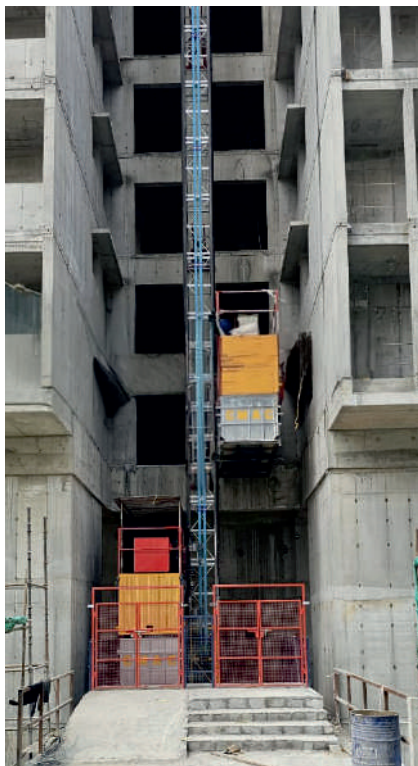
PM Hoist Double Cage
