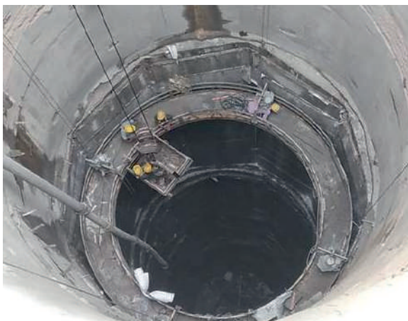
Vertical Duct Shaft at Kaleswaram
