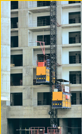
Passenger & Material Hoist (PMH)
