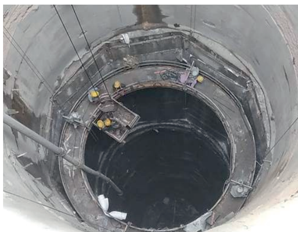
Vertical Duct Shaft at Kaleswaram
